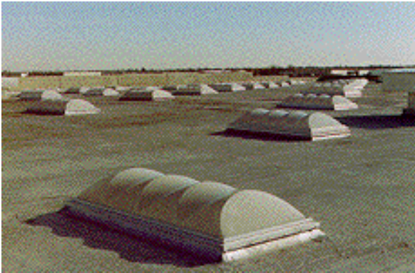
Figure 1: Compound parabolic skylight
